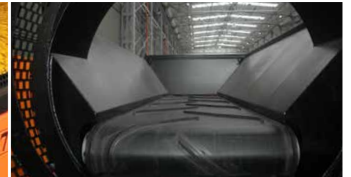
Reinforced belt on in-feed hopper conveyor
