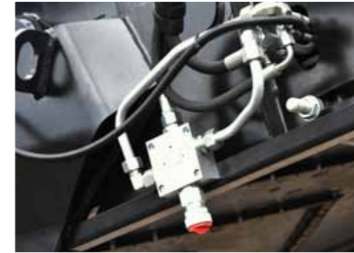
Conveyor belt speed rate adjustment
