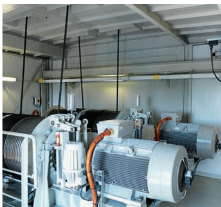
↑ Machinery room: spacious and maintenance-friendly
