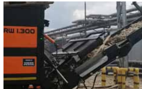
Magnetic separator for separating ferrous elements from shredding material
